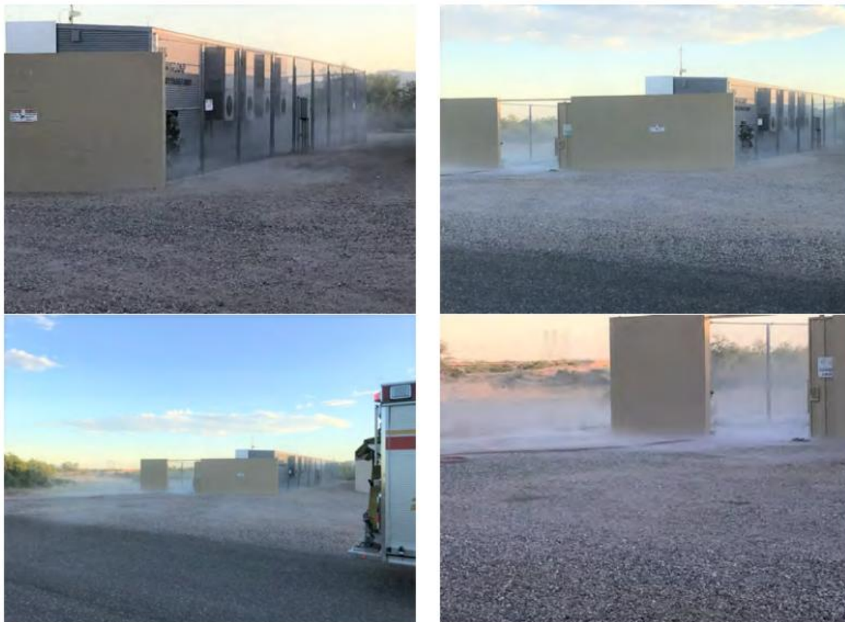
Figure 15 Photograph taken during the Surprise, AZ battery energy storage system incident, showing a white fog along the ground. Photograph from UL. 67
